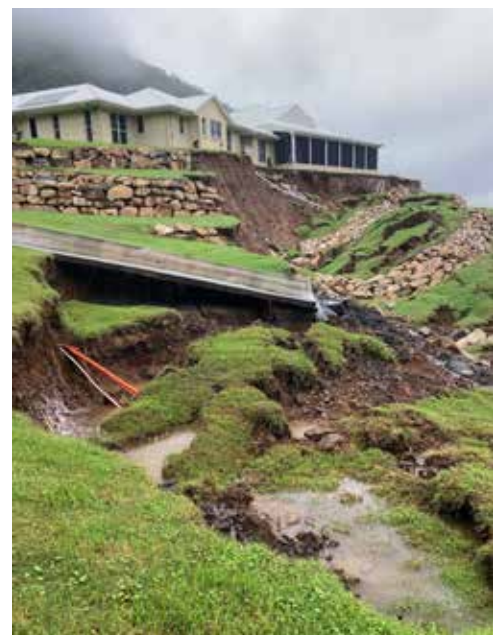
A landslide in Wongawallan. Photo by Robert Bloss.
