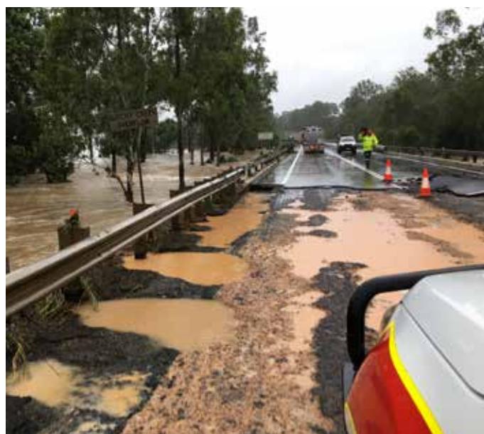
Floodwater caused extensive damage to roads.
