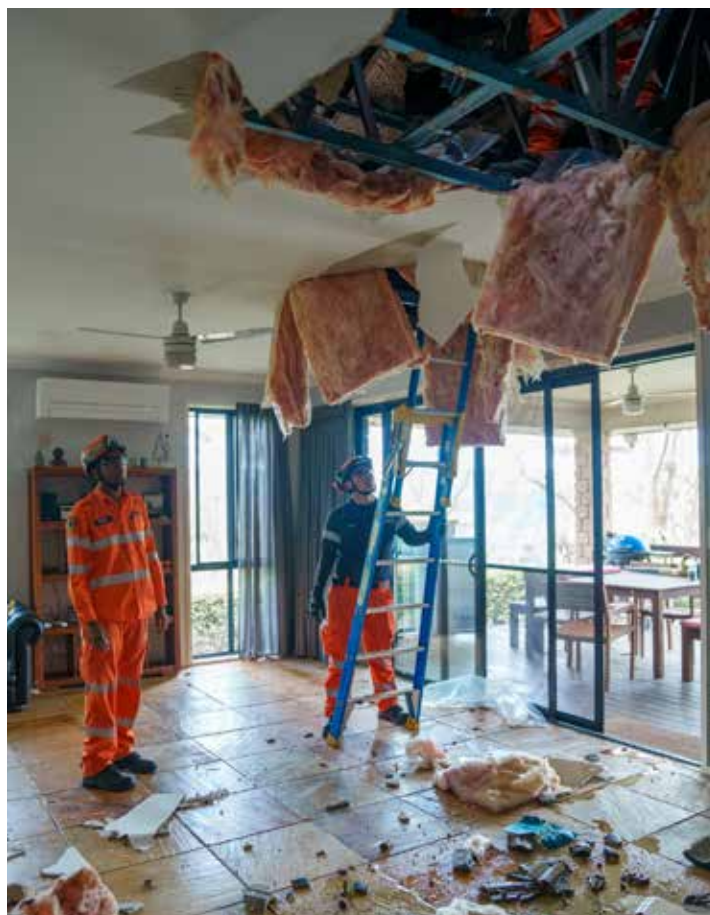
SES crews performed thousands of tasks helping people whose homes were damaged in the storms, like this home in Wongawallan.
