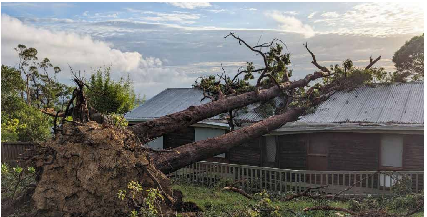
Travis Green's neighbourhood on Tamborine Mountain suffered extensive damage.
