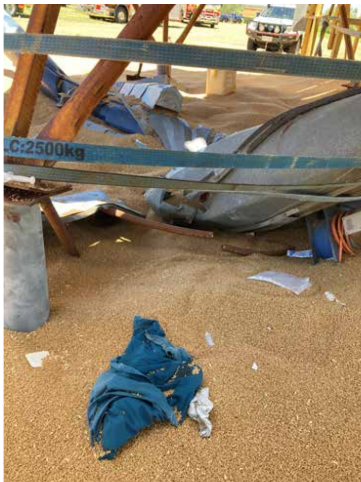
The man was dragged out from under this piece of metal.
